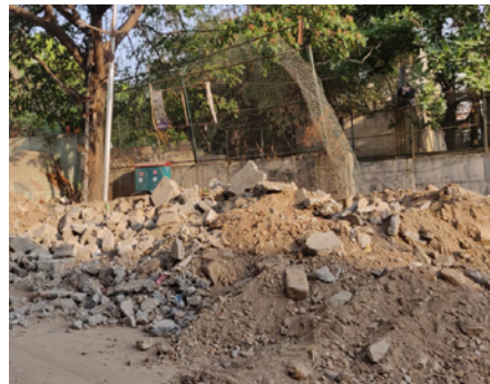
Construction Debris Sand and concrete waste Present around nearby construction sites
